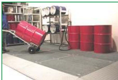
Ground protection basins 96-97
