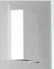
Air vents with fire protection
